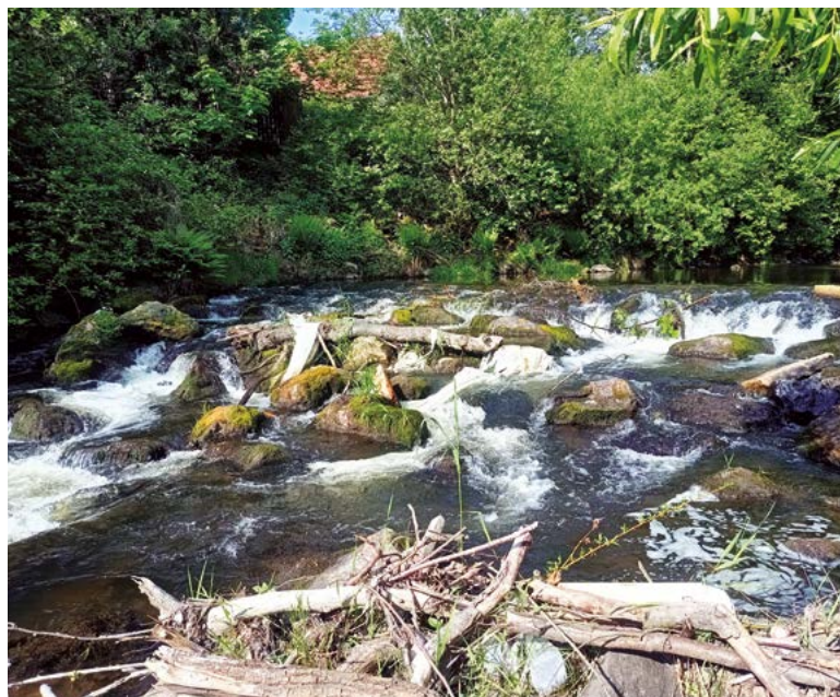
Fig. 5. Weir in Karlovy Vary at river km 1.5 – an example of a migration barrier with a damaged structure (photo: E. Bouše)
