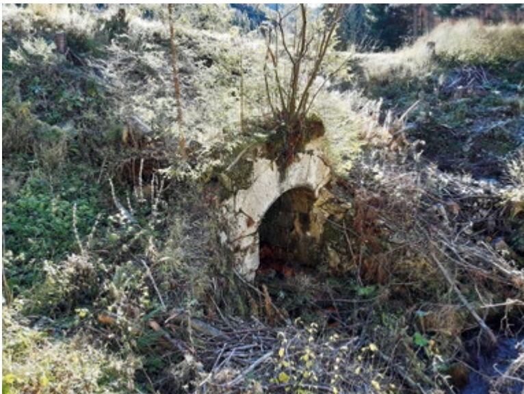
Fig. 9. Portal of a disused outlet gallery preserved in the embankment of Malužiná splash dam, November 2025
