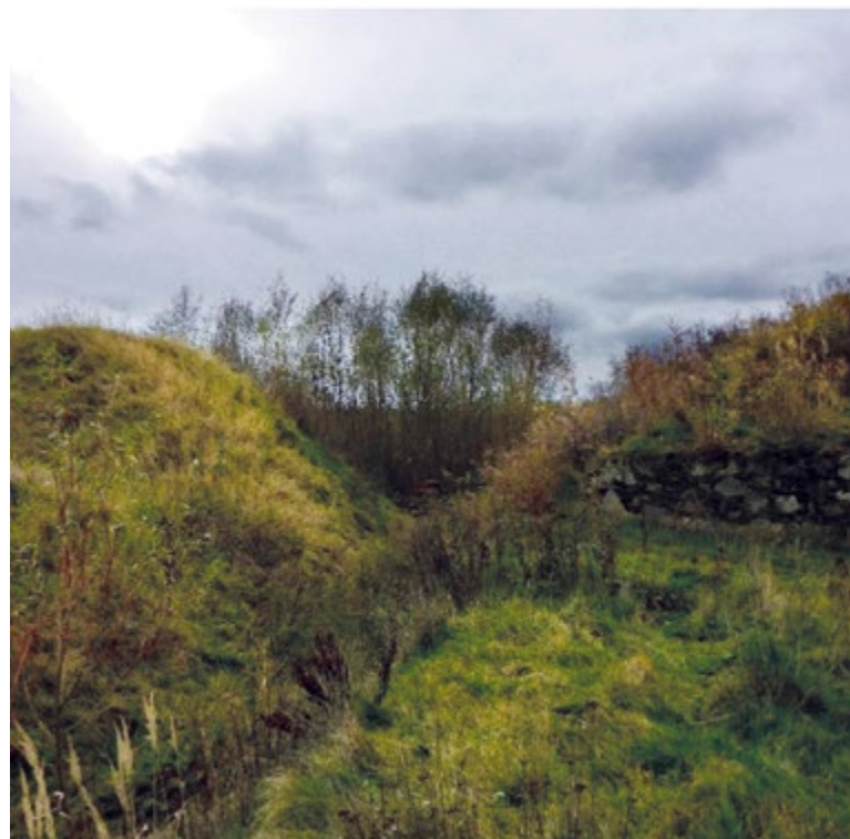
Fig. 6. The gap in Mlékovický Pond dam and the state of vegetation in the flooded area four years after the breach, as of 2017 [20]
