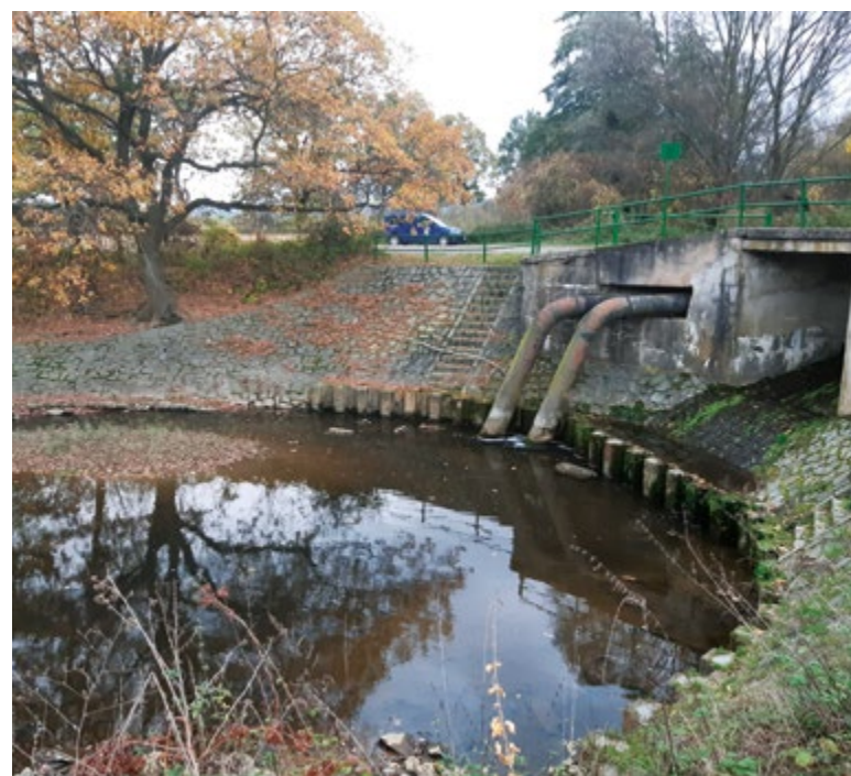
Fig. 8. Current situation below Bojmany weir at the spillway for the riverbed, which was used to supply the disappeared pond system and now returns behind the weir to the Doubrava river (November 2023)
