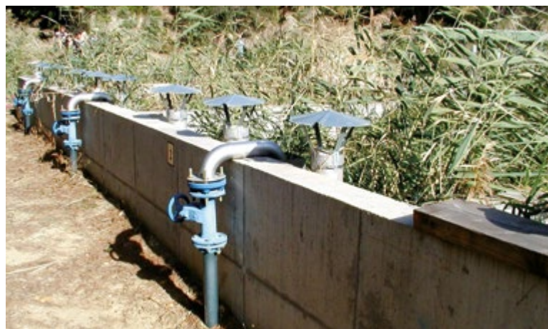
Fig. 1. STRB unit with controlled pipe system for filling and ventilation, larger WWTP with SBR reactor, France
