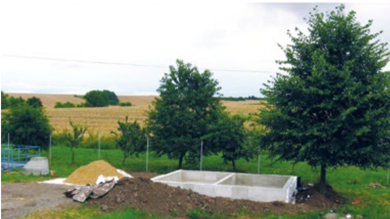
Fig. 3. An example of the construction of the basic structure of two STRB units to ensure the alternating operation of filling, dewatering, and stabilization of sludge from the settling tank of the constructed wetland, Czech Republic
