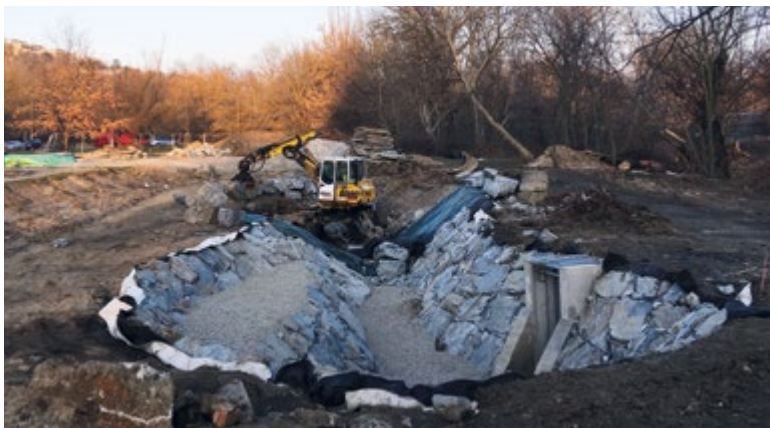
Fig. 4. Status of earthworks as of 1. March 2023 (view to the east, in the foreground is the future lake basin with an already established monk sluice)
