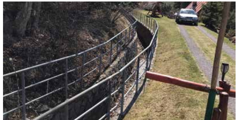
Fig. 9. Inappropriate reconstruction of one of the collecting ditches (Photo: S. Červeň)
