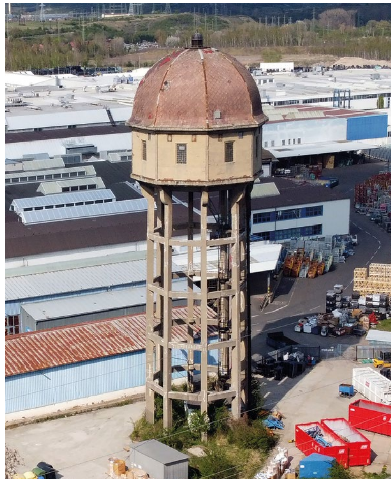
Fig. 12. The elevated water tank of the former glass factory in Bílina-Chudeřice is an example of the use of a subtle open reservoir-bearing structure (Photo: M. Postl)
