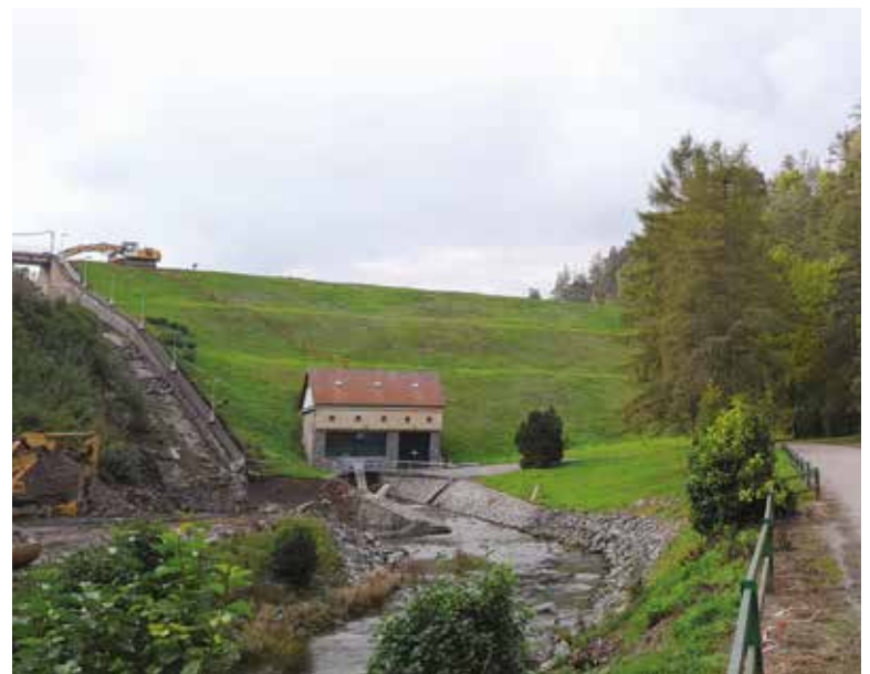
Fig. 7. Letovice hydraulic structure, an earth-filled dam completed in 1976. Its condition at the time of repairs of the safety spillway in 2022 (Photo: M. Forejtníková)
