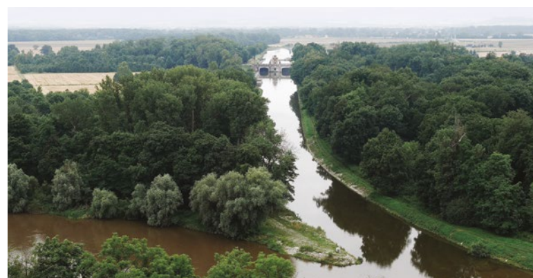
Fig. 8. Hořín lock, situation after modification of the right large lock chamber and replacement of the bridge over it (Photo: M. Ryšková, 2021)
