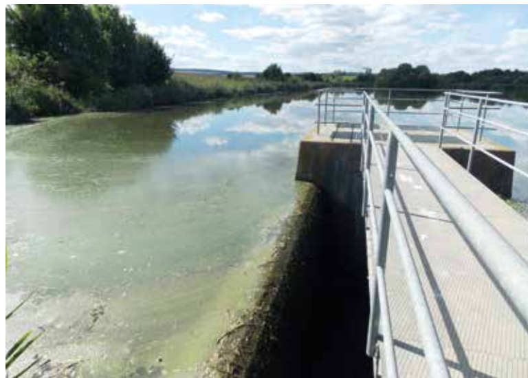
Fig. 9. Dry polder Želeč, referred to as a reservoir with flood protection purposed, but operated as fully filled (AQUATIS, a. s.)
