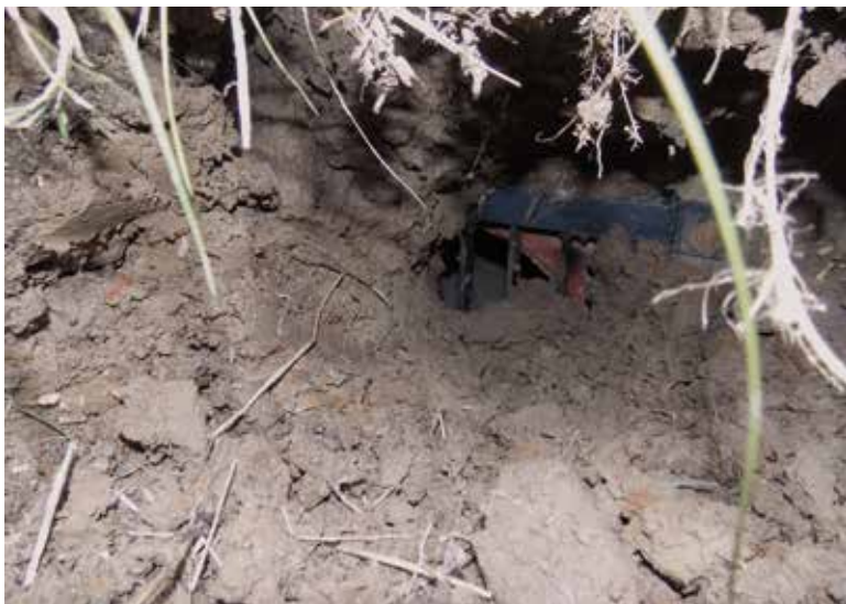
Fig. 7. Example of a completely clogged inlet part to the bottom outlet of the DR – Polder N5 (AQUATIS, a. s.)
