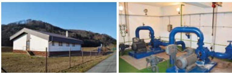
Fig. 7. Rapotín Water Treatment Plant with intake well (left), engine room (right) (March 2022, A. Létal)
