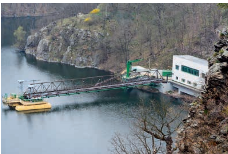
Fig. 6. Collection structure located on a floating pontoon
