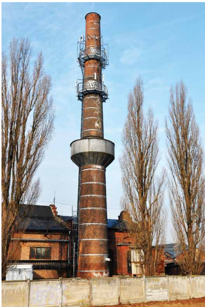
Obr. 6. Komín s vodojemem válcovny trub (2011) Fig. 6. The chimney with a water reservoir of the tube mill (2011)
